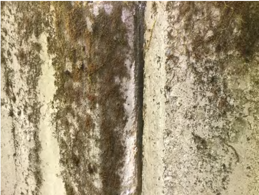
Another lockblock cracking
