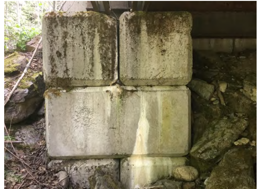
Downstream right bank lockblock cracked with efflorescence
